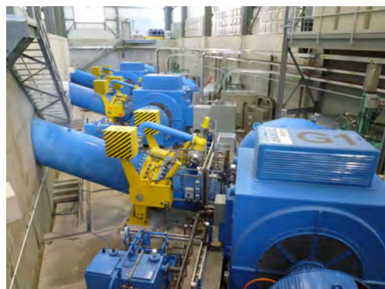
Picture 5 Electric generator
